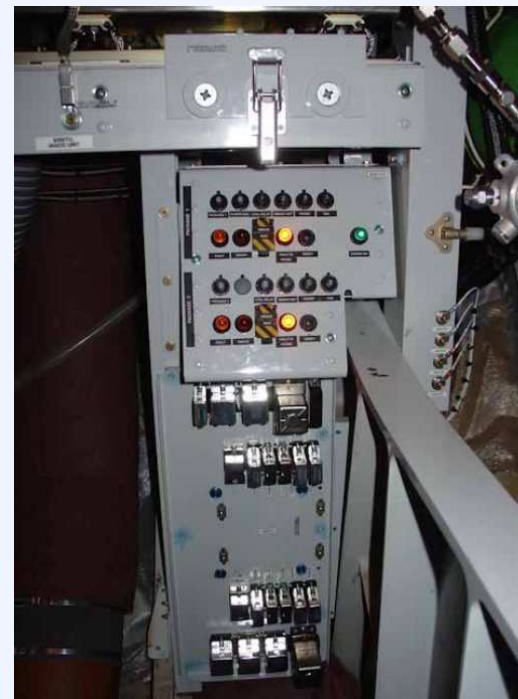
IAGOS Control Panel, Safety and test P/B
